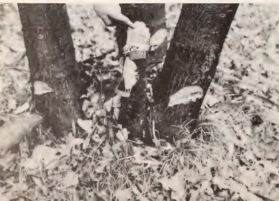
Figure 2.--Ammate crystals are placed in notches cut in large trees or in the tops of small stumps.
